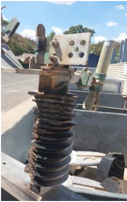
Figure 8: Cycloaliphatic polymer insulator affected by insulator pollution
