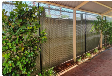
Plants on substation boundary must be kept trimmed
