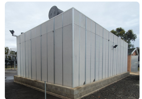
Acoustic barriers around equipment
