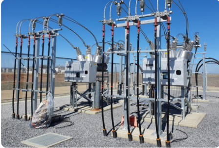
Substation yards kept neat and tidy
