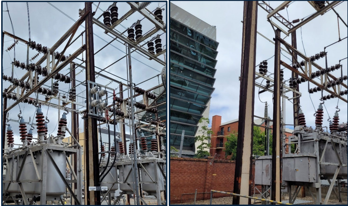
Figure 2: Bulk oil CBs below disconnectors (Left), and close proximity to CBD Street (Right)
