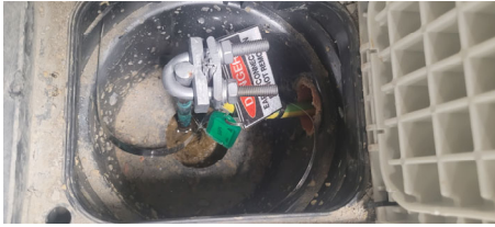
Figure 9 Earth connection in an earth stake pit
