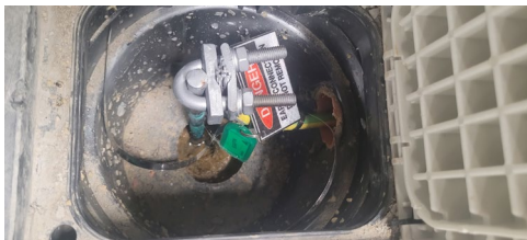
Figure 6: Earth connection in an earth stake pit
