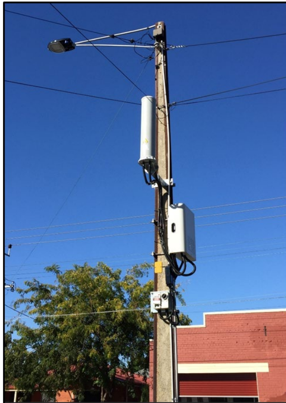
Figure 2: RF hazard warning sign Figure 3: Antenna with RF field warning hazard sign
