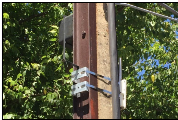
Figure 5: Stainless steel strapping arrangement on Stobie pole
