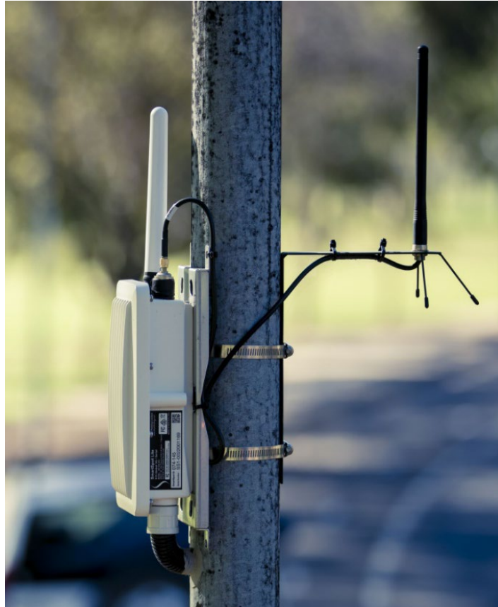
Figure 7: Stainless steel strapping arrangement on public light column
